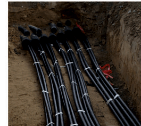
Underground Electric Network
