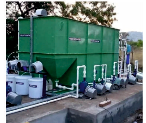
Sewage Treatment Plant
